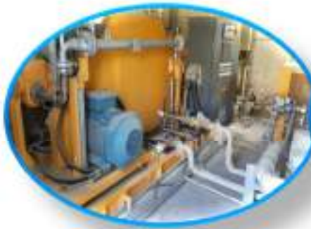
Compressed Air System
